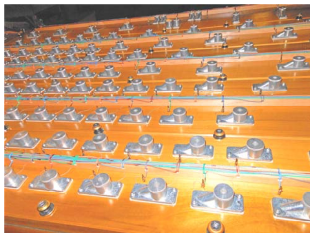
Bottom of a wind chest showing the electrical air release valves which operates the pallets on the other side on the side of the wind chest.
